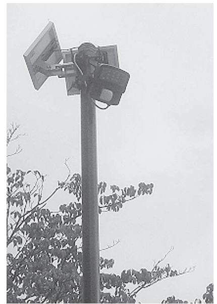
LED 避難誘導灯
